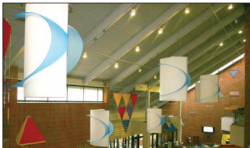
Recently installed high-efficiency lighting in East Campus Atrium will replace existing track lighting.
